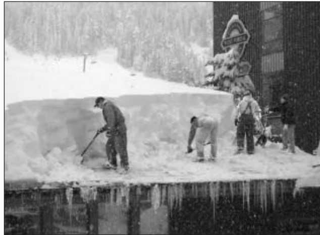
Workmen shoveling the roof of the Winter Park lodge on Wednesday, March 19th.
